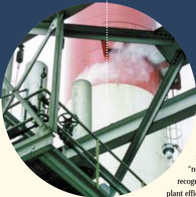
Main steam leaking from atmospheric vent valve.
