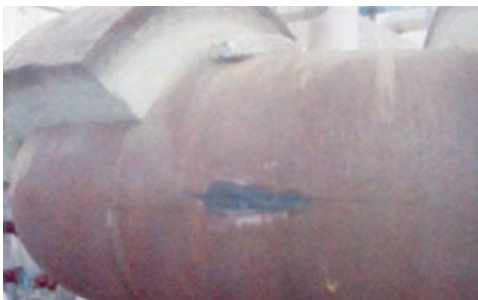
Figure 2: Illustrations of damage due to thermal cycling, often caused by poor attemperator performance.
